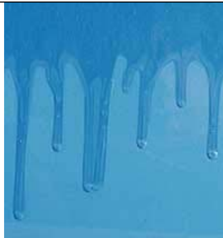
Figure 8. Example of excess flow paint on finished surface
