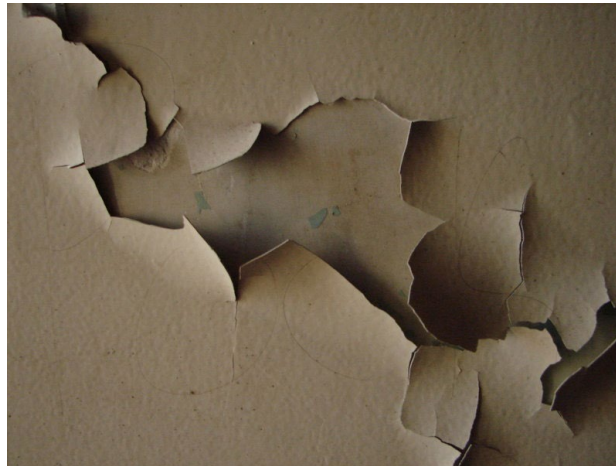
Figure 4-21 – Peeling, Flaking, Chipping
