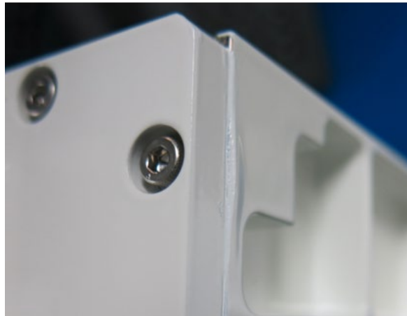
Figure 4-126 – Edge buildup - Excessive buildup/run at the edges (rejectable condition)
